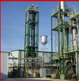
Process Plants: Supported by Intech
